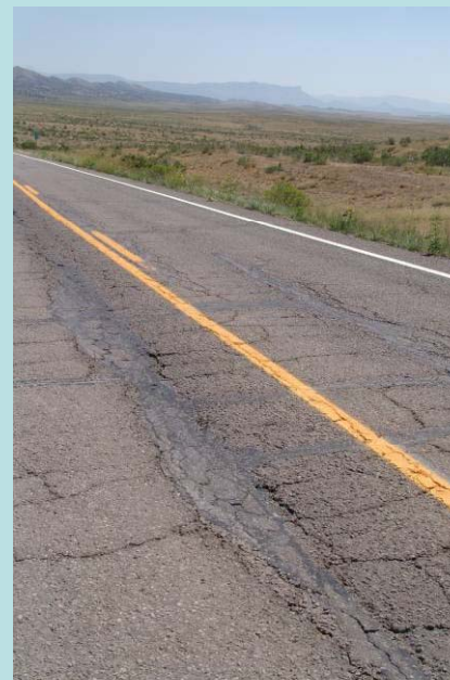
Cracking on SH 141
