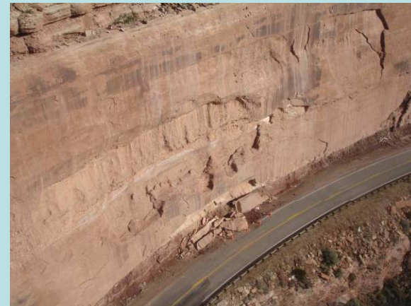
Rockfall on SH 141
